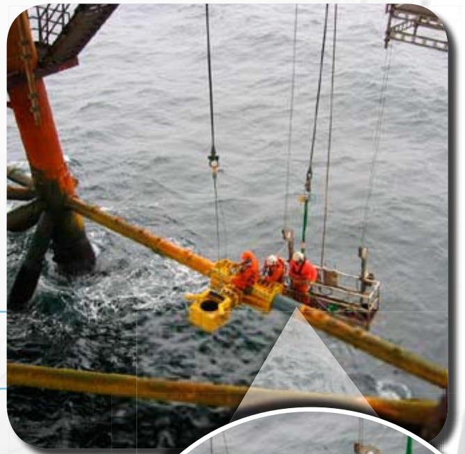
Air-driven ALTA platforms, offshore platform North Sea
