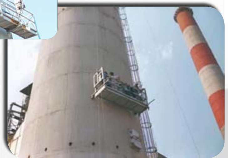
4 m ALTA platform on refinery stack, Thailand
