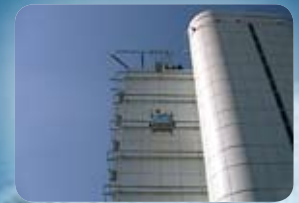
ALTA platform with monorail RAILSCAF, France
