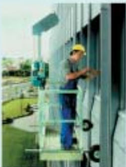
Access cradle for facade maintenance
