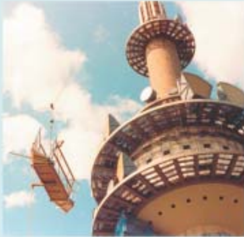
Lifting a component for a TIRAK® round platform using a return pulley block system.
