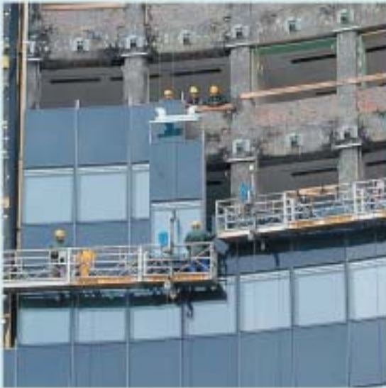
Facade assembly with lifting work platforms. Facade units are moved to the required position in the same way, using TIRAK® hoists.
