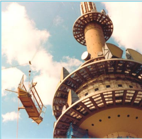
Lifting of a circular platform segment – tirak® at ground level, wire rope guiding by deflection pulley.
